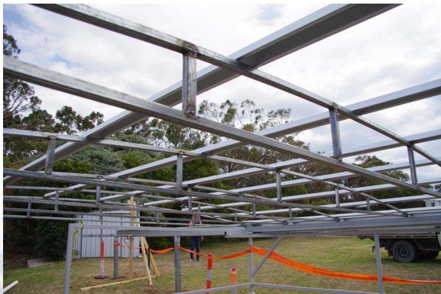
Above - Roof trusses made and bolted in place... then roof battens & bracing is tek-screwed in place.
